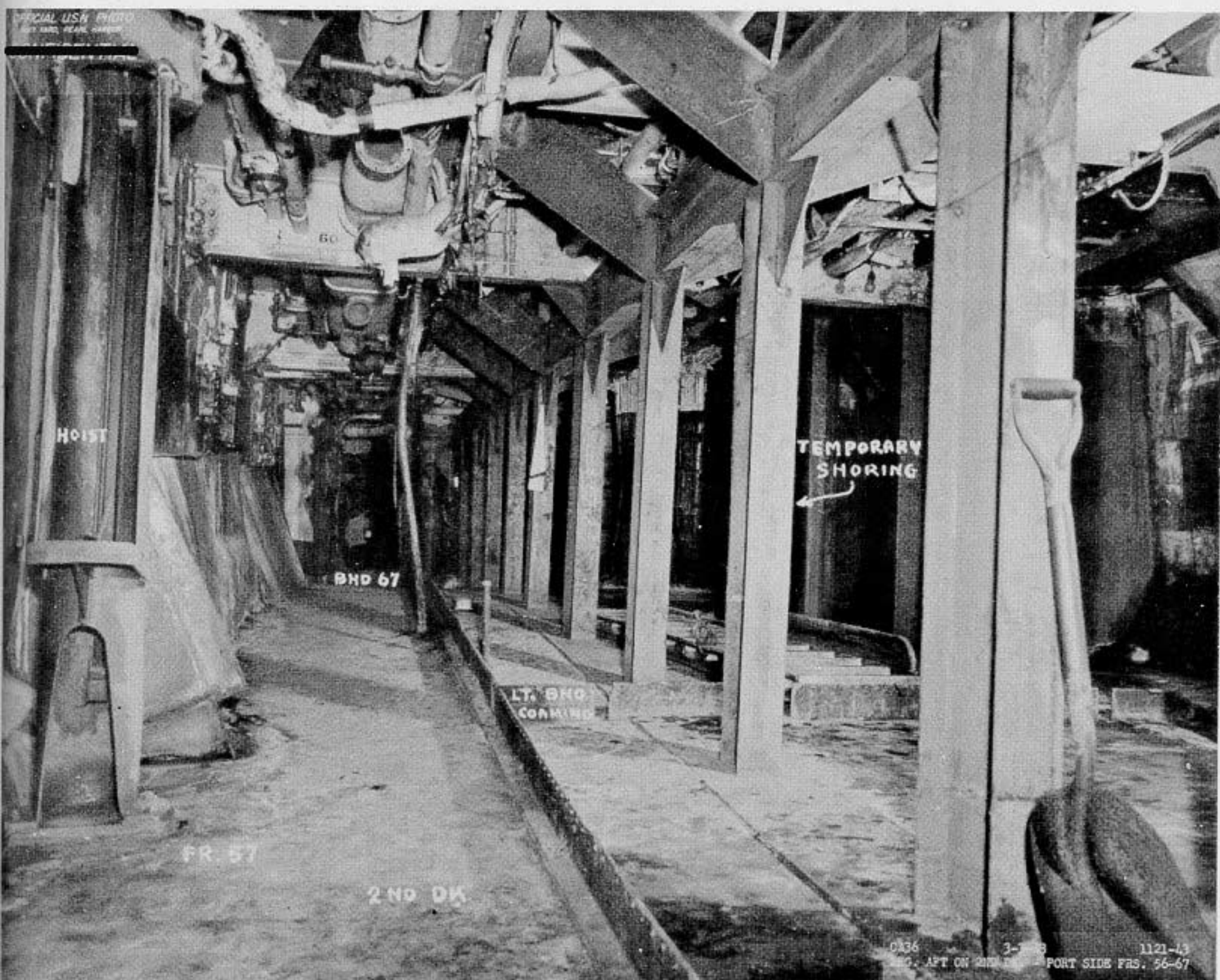
Photo No.26: USS MINNEAPOLIS - Port side second deck looking aft showing temporary shoring.
