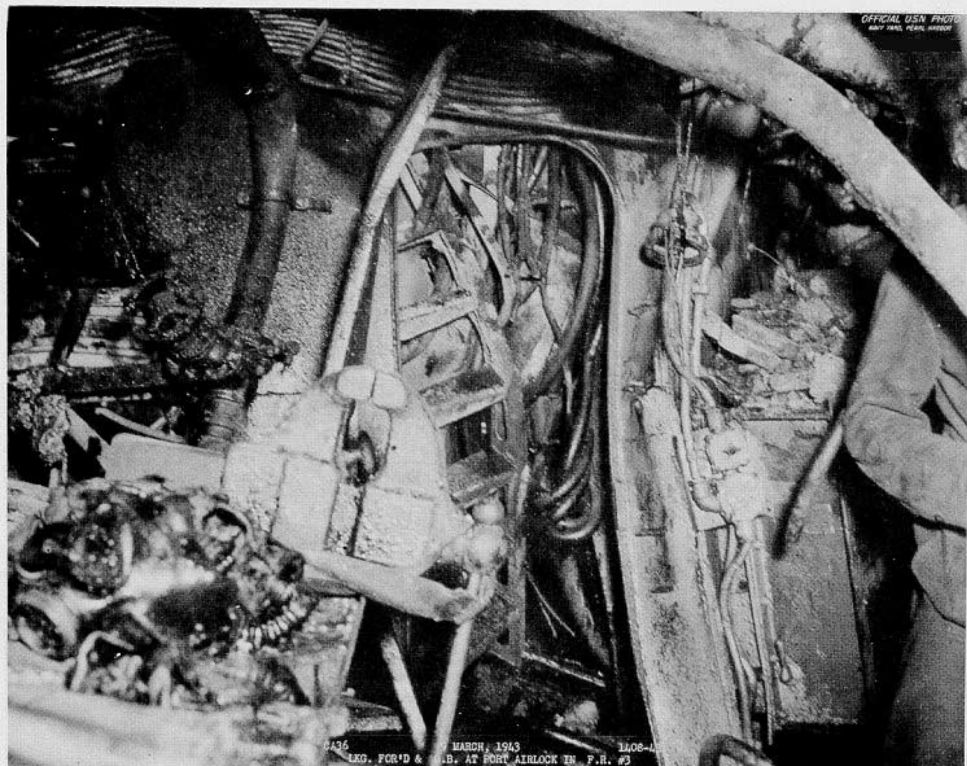
Photo No.24: USS MINNEAPOLIS - Port airlock in No. 3 fireroom looking forward and outboard.
